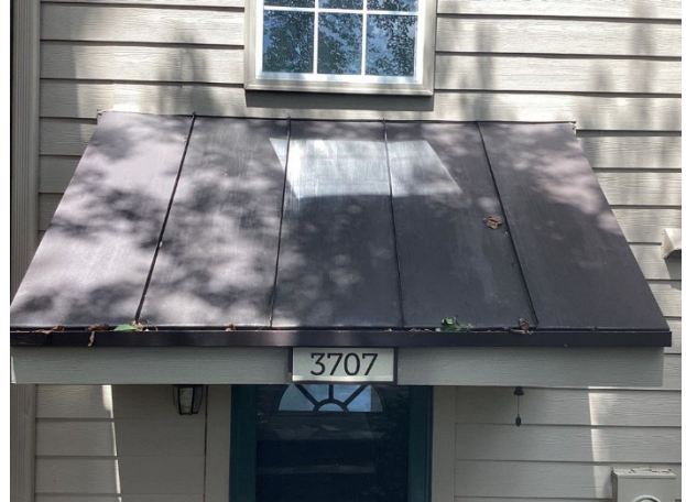
Metal roof finish deterioration
