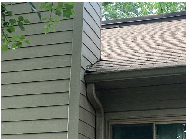
Siding deterioration evident
