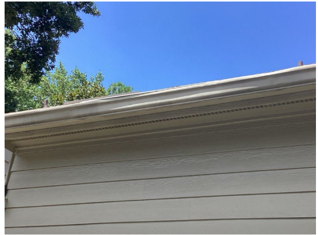
Damage at aluminum gutters
