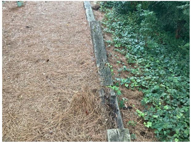
Timber retaining wall - wood rot and leaning sections evident
