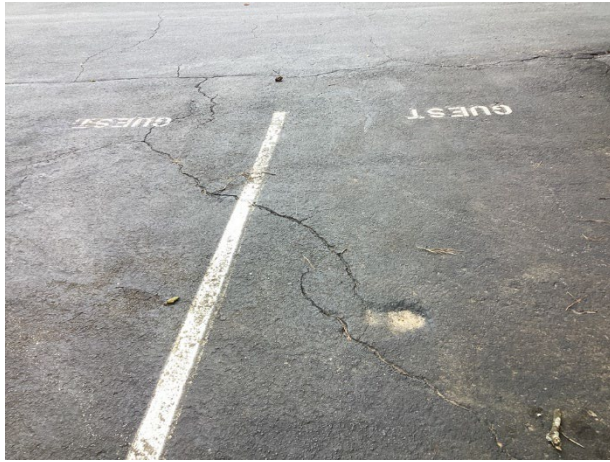
Pavement cracks near clubhouse
