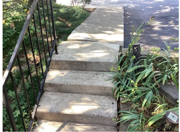
Sidewalk settlement at concrete steps
