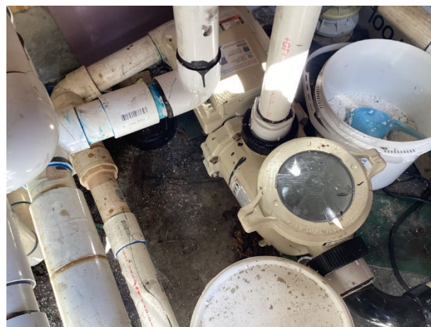
Pool mechanical equipment
