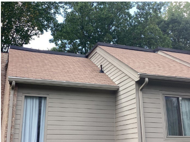
Roof overview - shingle curl and sheathing deflection evident
