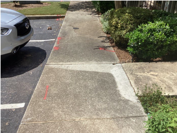
Concrete sidewalk - cracks and previous repairs evident
