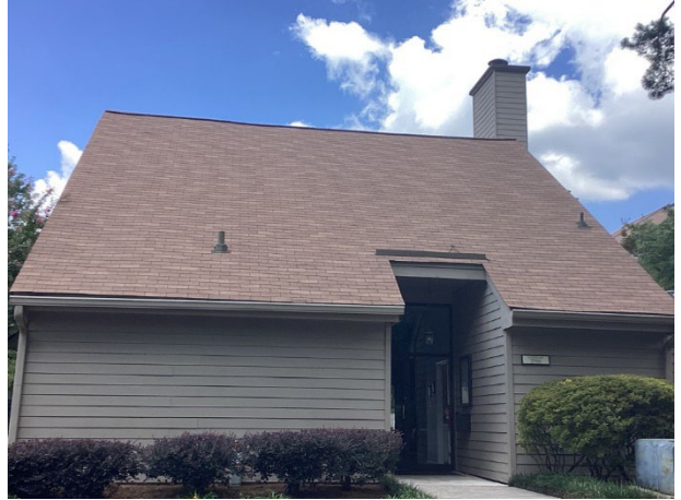
Clubhouse roof - shingle curl and sheathing deflection evident
