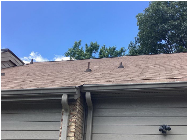
Penetrations at townhomes
