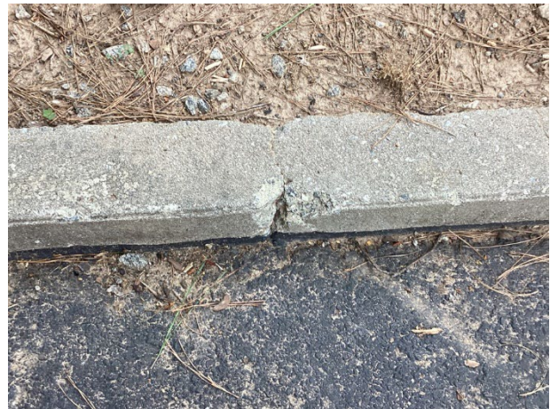
Concrete spalls and cracks
