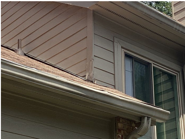
Wood trim deterioration
