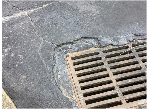
Pavement overlay evident
