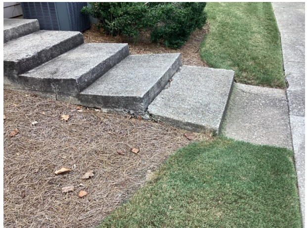
Sidewalk settlement at concrete steps
