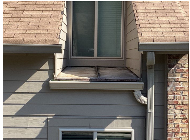
Metal roof deterioration evident
