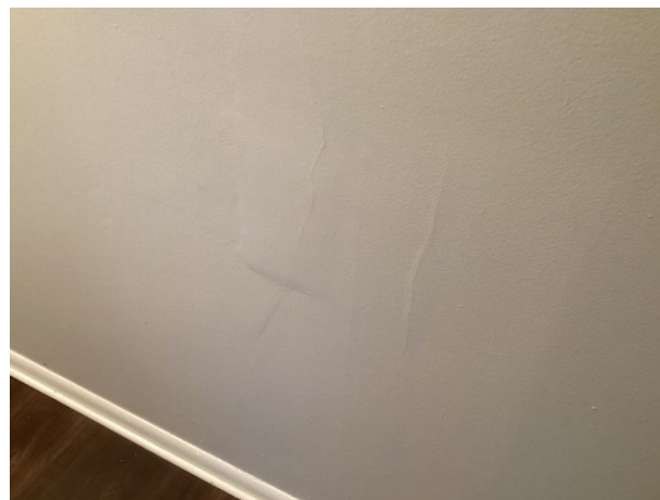
Paint finish deterioration
