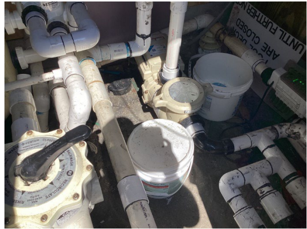
Pool mechanical equipment
