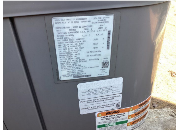
Condensing unit details
