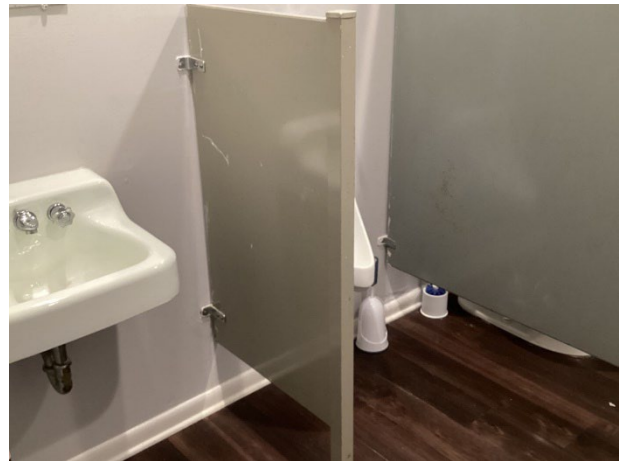
Partition finish deterioration
